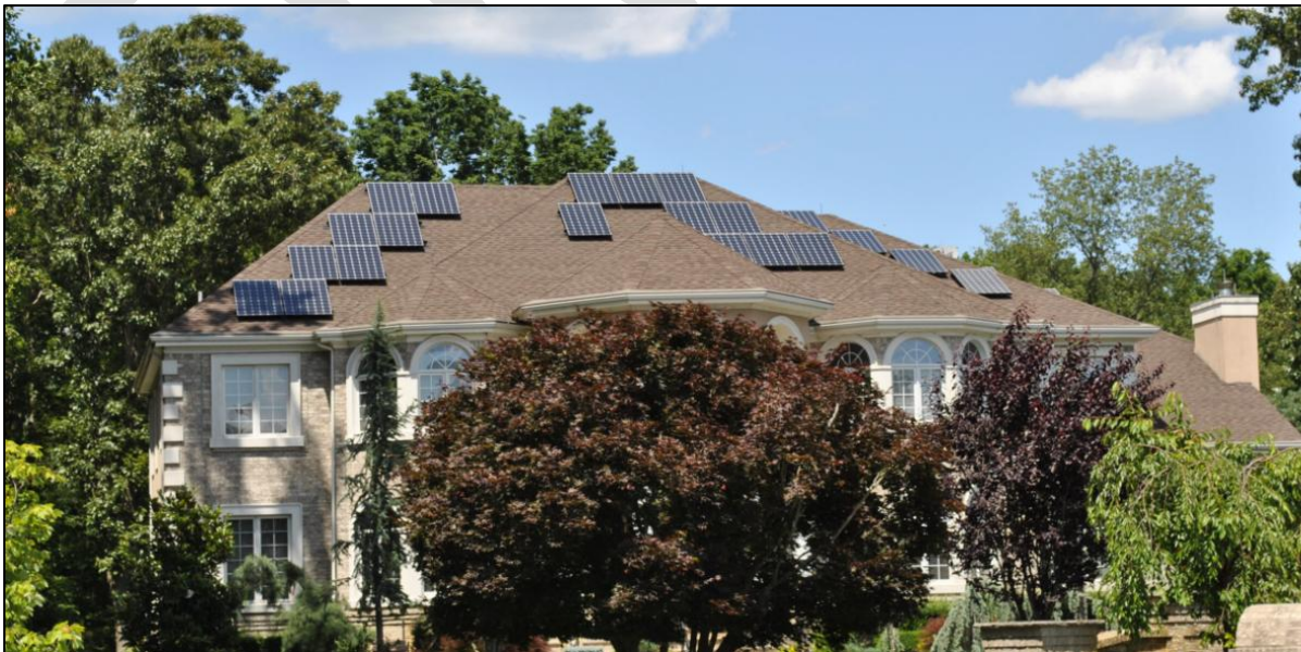
A disjointed arrangement of panels, some configured in a stair-step pattern.
