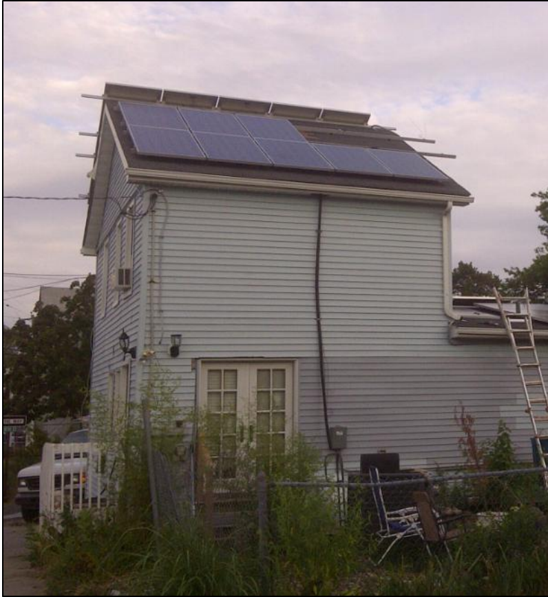
Panels and mounting rails extend beyond the roof. Panel-related equipment is not colored to match the surface to which it is attached.
